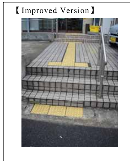
Fig. 70: Warning blocks should generally be installed at the top of stairways and on the ground or floor following the final step. Here, the warning blocks at the bottom of the stairs have been installed not on the ground level but on the final step. People with impaired vision coming down the stairs will sense the warning blocks and determine that they have reached ground level. Because in fact they have an additional step to go, this may lead to accidents such as falls or twisted ankles. Warning blocks should be repositioned as in the improved version. ( Aichi, Japan )
