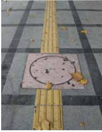
Fig. 30: Directional Blocks Interrupted by Manhole Cover (Seoul, Korea)
