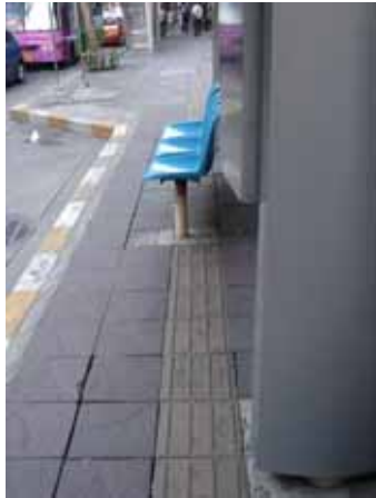
Fig. 102: Benches located above Tactile ground surface indicators at a bus stop in Thailand. (Bangkok, Thailand)
