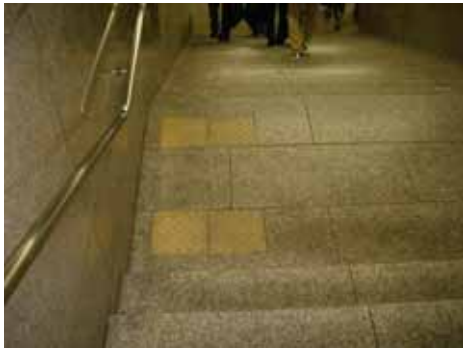
Fig. 74: In general, single rows of warning blocks should be installed at the beginning and end of stair landings. It is inappropriate to install them only near handrails rather than across the entire width of the stairs, as shown here. The elderly are the primary users of handrails at rail stations. Because of the danger of collision with the elderly, many people with impaired vision do not use handrails when ascending and descending stairs. ( Osaka, Japan )
