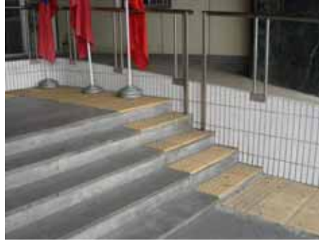
Fig. 71: Warning blocks are sometimes installed on each step of a stairway. Such warning blocks are unnecessary. (Taipei, Taiwan)
