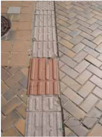
Fig. 99: The use of blocks different than those originally installed is common when Tactile ground surface indicators are repaired. The resulting mix of different specifications and shapes can lead to confusion among people with impaired vision. The loss of visual consistency is also unattractive. ( Fukuoka, Japan )
