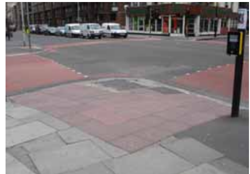
Fig. 62: Covering the sidewalk with blocks as in this example makes it impossible for users to determine where the crosswalks are or which direction to proceed. (London, UK)
