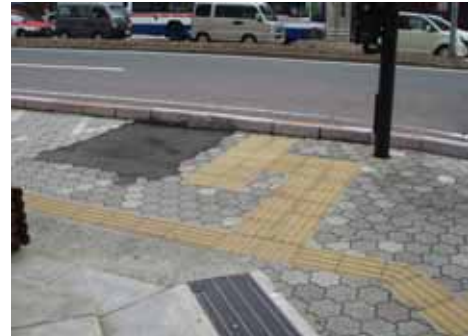
Fig. 92: The area filled in with black asphalt once contained some kind of equipment—probably a public telephone—yet the Tactile ground surface indicators were left as they were even after this equipment was removed. Such blocks should be adjusted when this kind of equipment is removed. ( Nagasaki, Japan )
