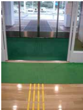
Fig. 104: Doormats designed to keep out mud sometimes cover Tactile ground surface indicators at building entrances. Such mats make it difficult to feel the protrusions on the blocks, however, and should not be used in this way. (Hokkaido, Japan)
