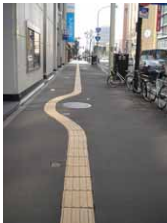
Fig. 36: Rerouting directional blocks to avoid the manhole, as in this photograph, not only looks unattractive but creates a winding course that greatly reduces the walking speed of people with impaired vision. ( Hokkaido, Japan )
