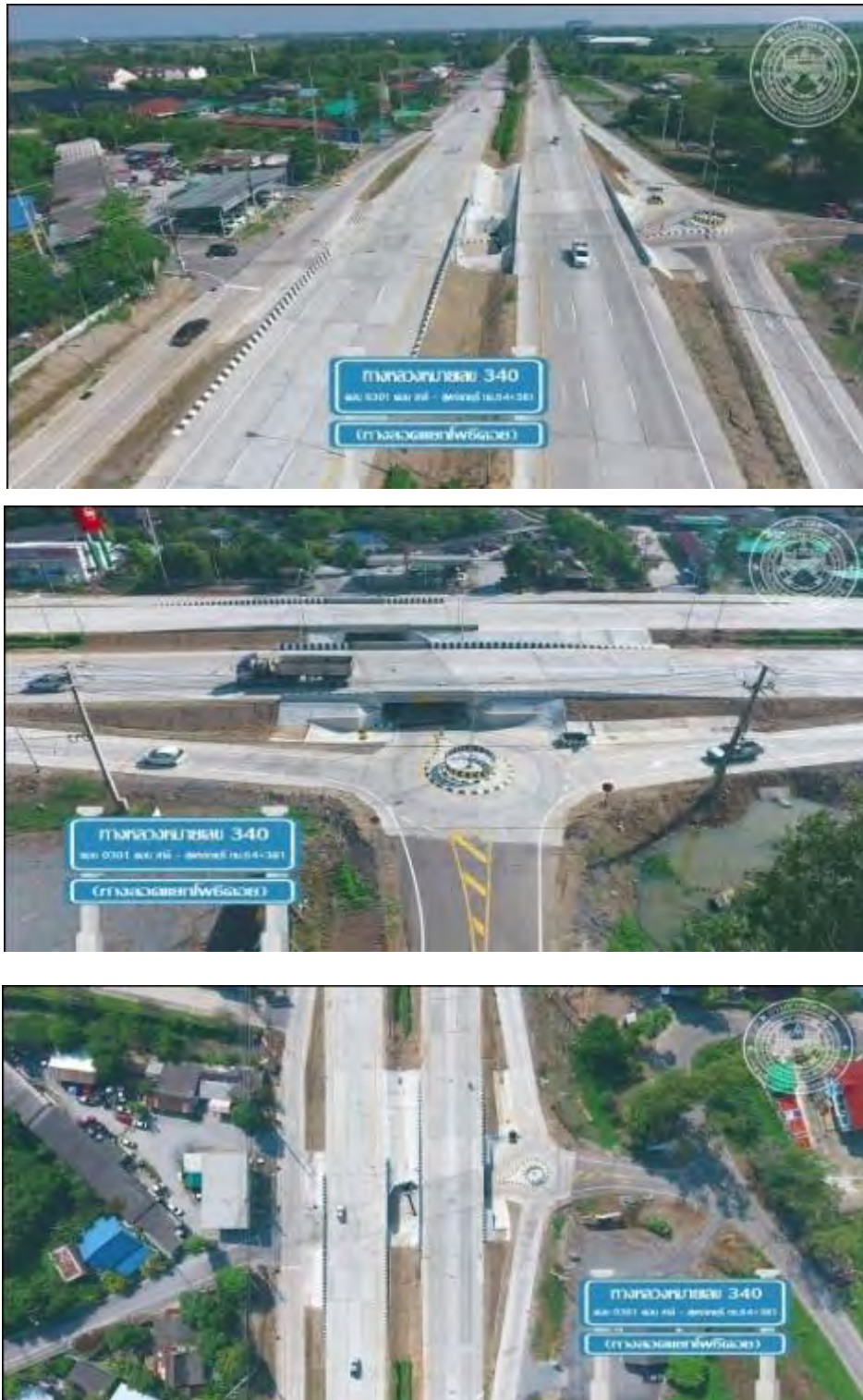
รูปที่ 8-21 The photos after the construction was completed according to the plan
