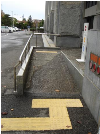
Fig. 83: Blocks are often installed at the beginning and end of slopes, but this creates a barrier for wheelchair users. (Ehime, Japan)
