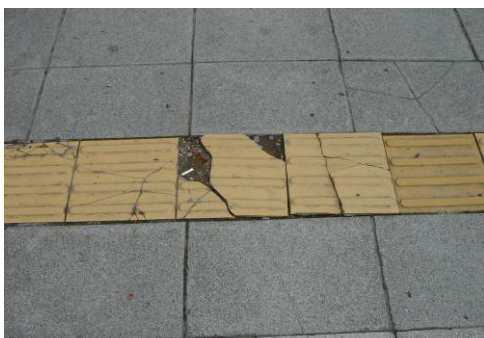
Fig. 96: An example of broken blocks left unattended. (Seoul, Korea)
