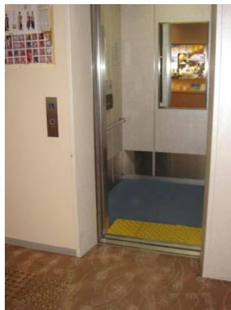
Fig. 86: Warning blocks are sometimes installed inside elevators. People with impaired vision, however, will not lose track of the entrance within the narrow confines of an elevator. Such blocks are an obstacle to wheelchair use and should be removed. (Ehime, Japan)
