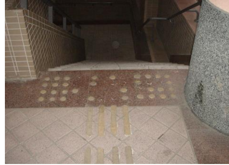
Fig. 95: Because the protrusions have disappeared from these warning blocks at the top of the stairs, people with impaired vision may not realize that there is a stairs and fall down. (Taipei, Taiwan)
