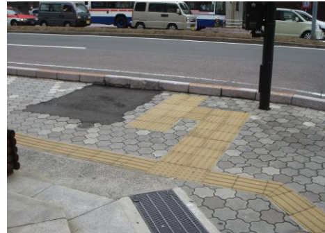
Fig. 92: The area filled in with black asphalt once contained some kind of equipment—probably a public telephone—yet the Tactile ground surface indicators were left as they were even after this equipment was removed. Such blocks should be adjusted when this kind of equipment is removed. (Nagasaki, Japan)
