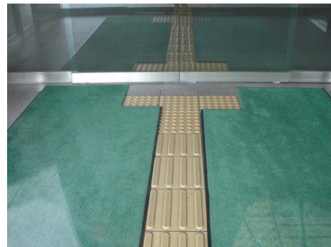
Fig. 105: Rather than cover the Tactile ground surface indicators with the mats, the mats should be shaped as shown to leave the blocks uncovered. (Hiroshima, Japan)
