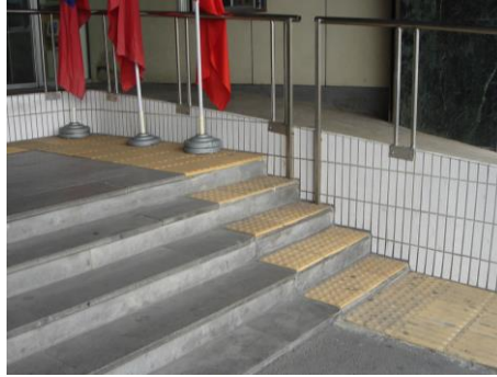
Fig. 71: Warning blocks are sometimes installed on each step of a stairway. Such warning blocks are unnecessary. (Taipei, Taiwan)
