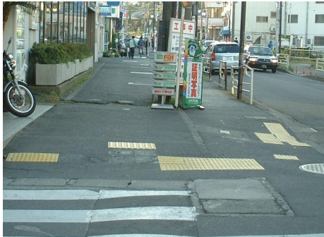
Fig. 94: Because the Tactile ground surface indicators have peeled away before the crosswalk, people with impaired vision may not recognize that there is a crosswalk and step out into the road. (Kanagawa, Japan)
