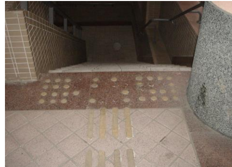
Fig. 95: Because the protrusions have disappeared from these warning blocks at the top of the stairs, people with impaired vision may not realize that there is a stairs and fall down. (Taipei, Taiwan)
