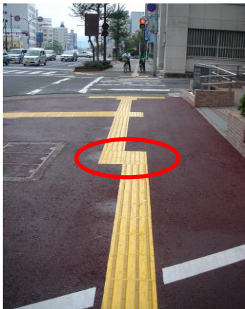
Fig. 51: Here, warning blocks have been installed where the row of directional blocks was shifted over to the left by the width of one block (30cm) before a crosswalk to align the directional blocks with the center of the crosswalk. As long as the directional blocks leading to a crosswalk are not too close to the crosswalk's edge, there is no need to install warning blocks and alter the course of the directional blocks in this way. (Hokkaido, Japan)
