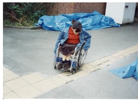
Fig. 97: Broken blocks not only pose a danger to people with impaired vision but are also a major barrier for wheelchair users.
