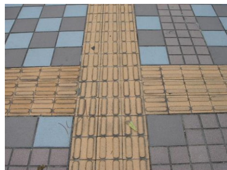
Fig. 27: Failure to Install Warning Blocks Where Directional Blocks Intersect (Taipei, Taiwan)
