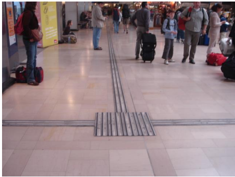
Fig. 7: Tactile Ground Surface Indicators at Montparnasse Station (Paris, France)
